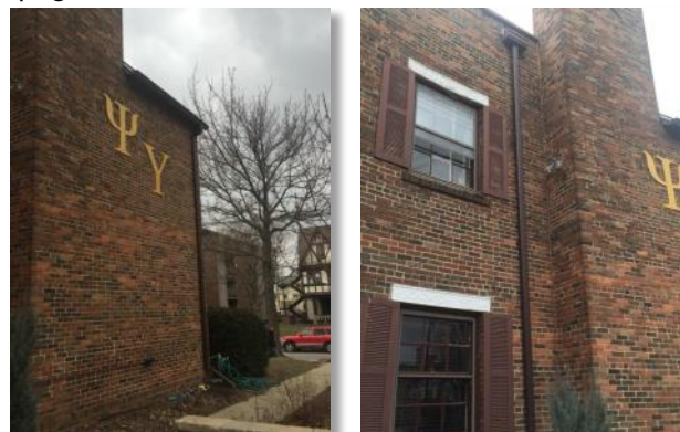
New guttering will allow for better preservation of brick, mortar, and interior plaster work
